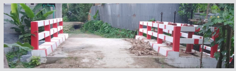
LGED at Dhamrai
